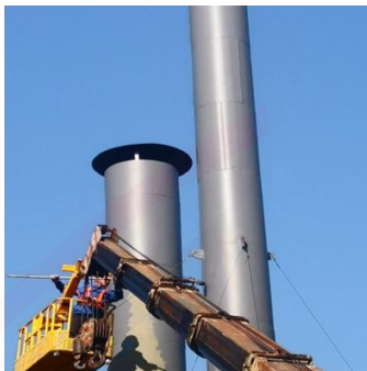
金德利摩擦片工厂排气管防腐, 绍兴, 浙江 Jindeli Friction Plate Factory Exhaust Pipe Anti-corrosion, Shaoxing, Zhejiang
