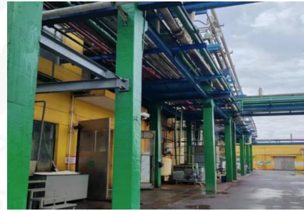
海昇药业厂区管道架防腐, 衢州, 浙江 Haisheng Pharmaceutical Factory Pipeline Rack Anti-corrosion, Quzhou, Zhejiang
