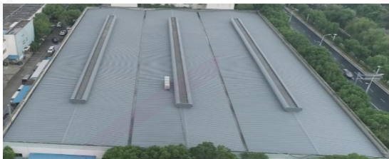
苏州奥星电子厂房彩钢瓦屋顶防腐工程，苏州，江苏 Suzhou Aoxing Electronics Factory Color Steel Tile Roof Anti-corrosion Project, Suzhou, Jiangsu
