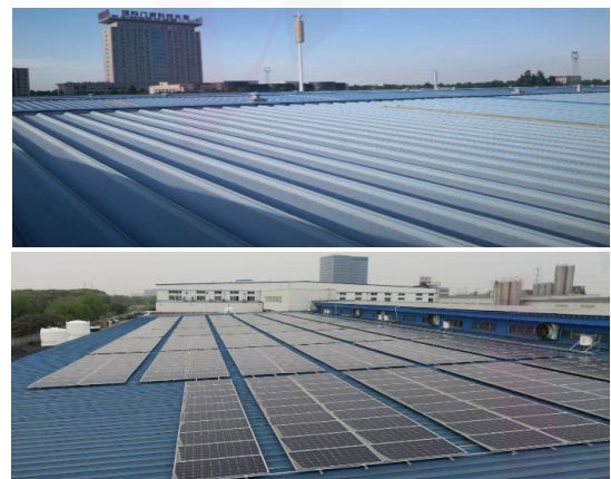
河北奥润顺达工厂彩钢瓦屋顶防腐工程，高碑店，河北 Hebei Aorun Shunda Factory Color Steel Tile Roof Anti-corrosion Project, Gaobeidian, Hebei
