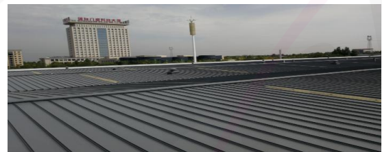
大同电工工厂彩钢瓦屋顶防腐工程，苏州，江苏 Datong Electric Factory Color Steel Tile Roof Anti-corrosion Project, Suzhou, Jiangsu
