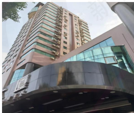
龙宝大厦砖结构外墙防水装饰，北京 Longbao Building (Brick Structure Exterior Wall), Exterior Wall Waterproof&&Decoration, Beijing
