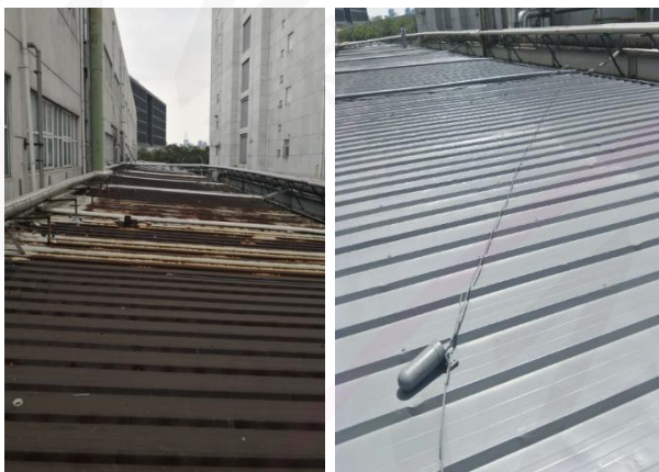
正泰新能源工厂彩钢瓦屋顶防腐工程，杭州，浙江 New Energy Factory Color Steel Tile Roof Anti-corrosion Project, Hangzhou, Zhejiang
