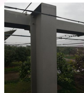
椒江区污水厂钢结构防腐, 台州, 浙江 Jiaojiang District Sewage Treatment Plant Steel Structure Anti-corrosion, Taizhou, Zhejiang
